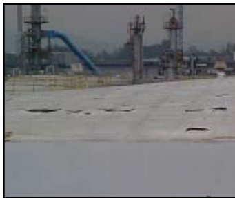
HOLES IN THE ROOF OF AN AST
