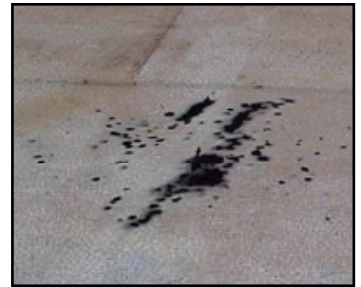
A CLOSE VIEW OF HOLES IN THE ROOF OF AN AST
